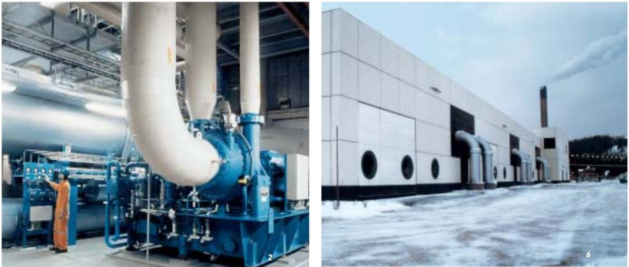
Figure 16: General view of an HP unit (left) and the machine room building (right) [10]
