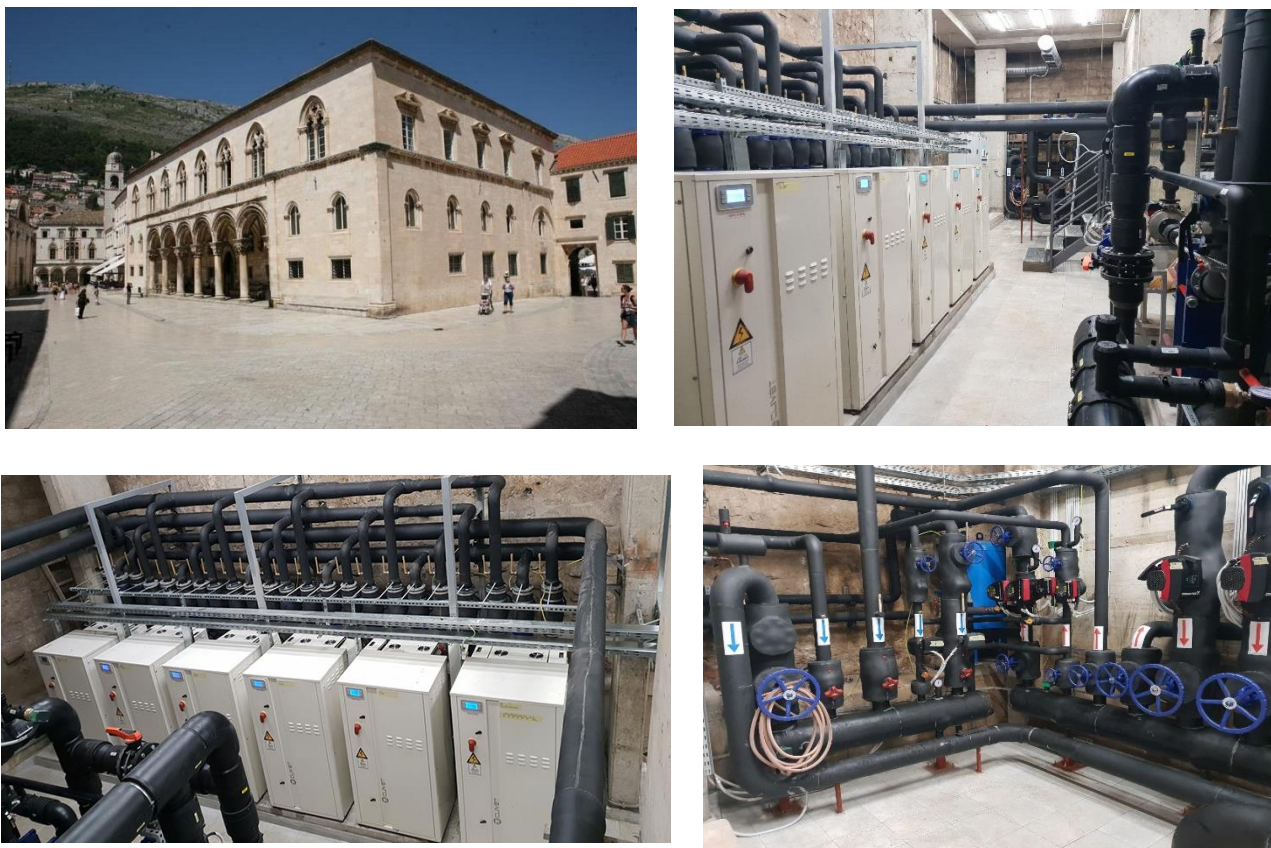
Figure 15: Seawater heat pump system in the historical town of Dubrovnik
